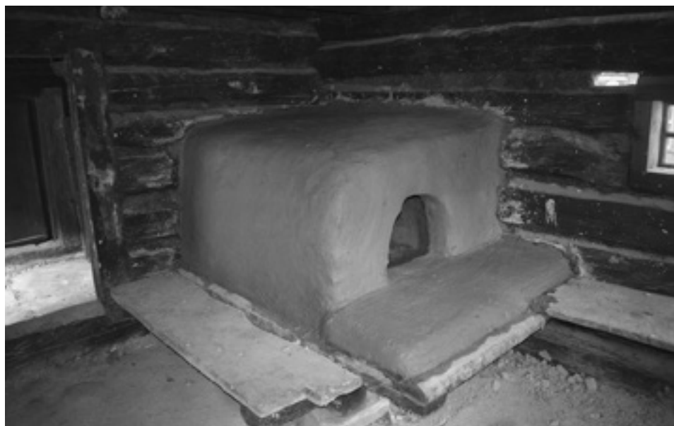
Obr. 3. Opravené vykurovacie zariadenie v dome zo Štiavnika. Foto J. Neplech, 2019 Fig. 3. Repaired heating apparatus in the house from Štiavnik. Photograph by J. Neplech, 2019
